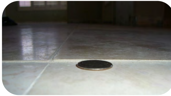
LIPPAGE (UNEVEN TILES)
