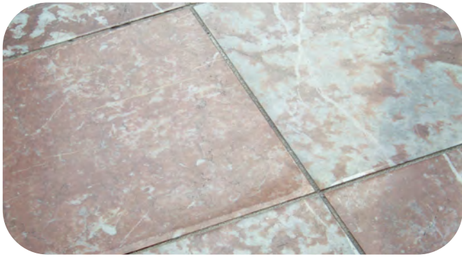
DIRTY, STAINED GROUT LINES
