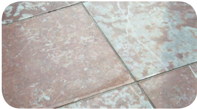
DIRTY, STAINED GROUT LINES
