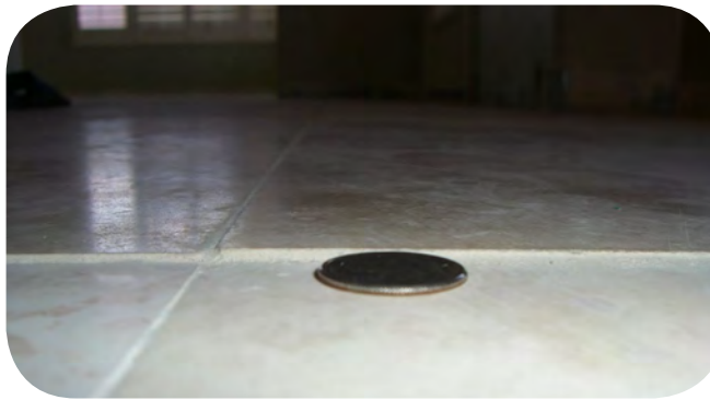
LIPPAGE (UNEVEN TILES)
