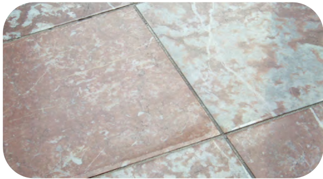
DIRTY, STAINED GROUT LINES
