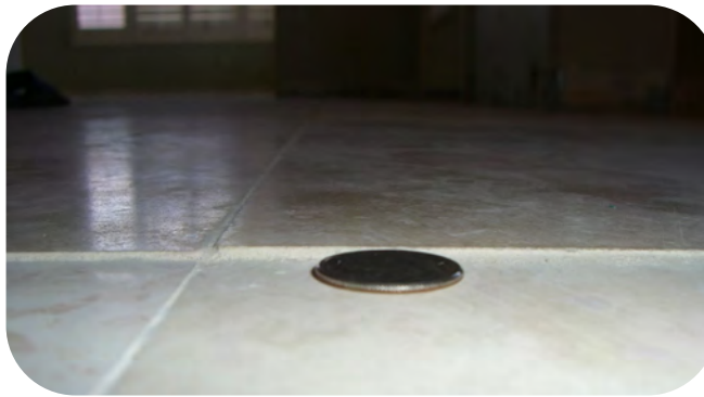
LIPPAGE (UNEVEN TILES)
